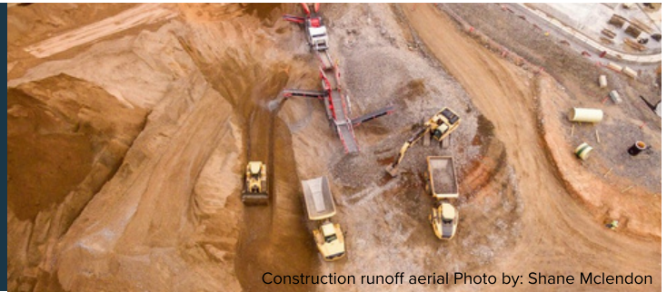
Construction runoff aerial Photo by: Shane McLendon
