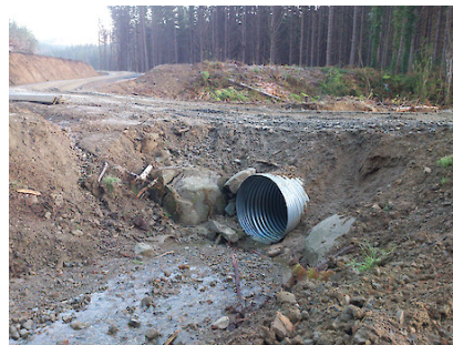
Pipe culvert. Photo credit: docs.nzfoa.org.nz
