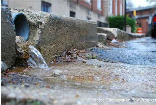
Stormwater entering the street
