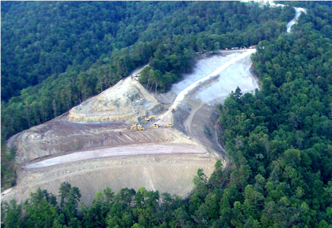
WELL PAD GRADING: SITE PREPARATION FOR STONE ENERGY BOYERS WELLPAD NEAR NEW MARTINSVILLE
