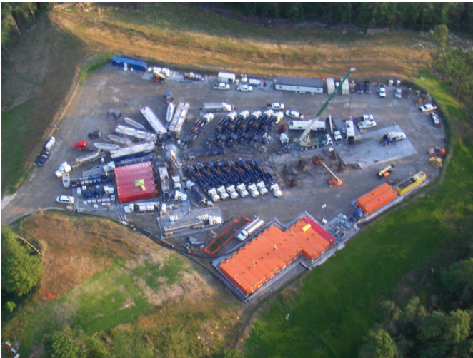
HYDRAULIC FRACTURING IN PROGRESS: STONE ENERGY'S BOWYERS WELL PAD IN WETZEL COUNTY, WV
