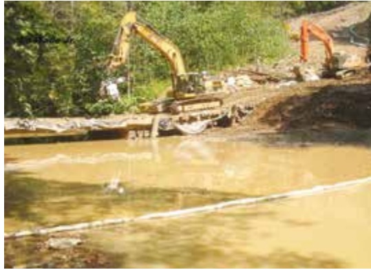
Sediment pollution caused by pipeline construction in West Virginia; photo courtesy Ed Wade, Jr.
